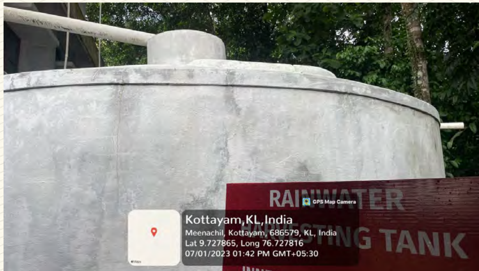
Figure 8: Rain Water harvesting tank Photo 1
