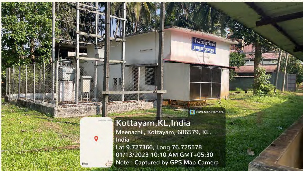
Figure 119: 11KV Substation photo 1
