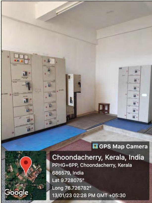
Figure 153: Electrical Circuit Room photo 1
