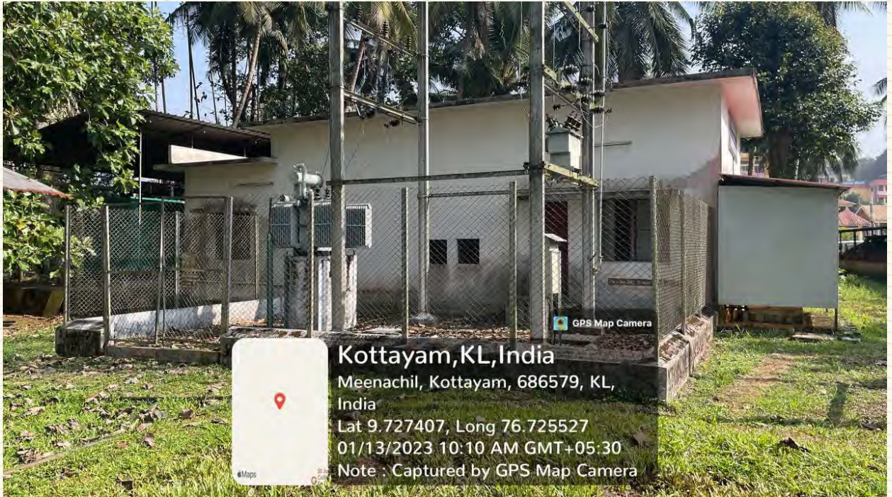
Figure 120: 11KV Substation photo 2
