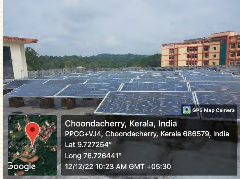
Figure 149:Solar Power Plant-roof top-20kWp
