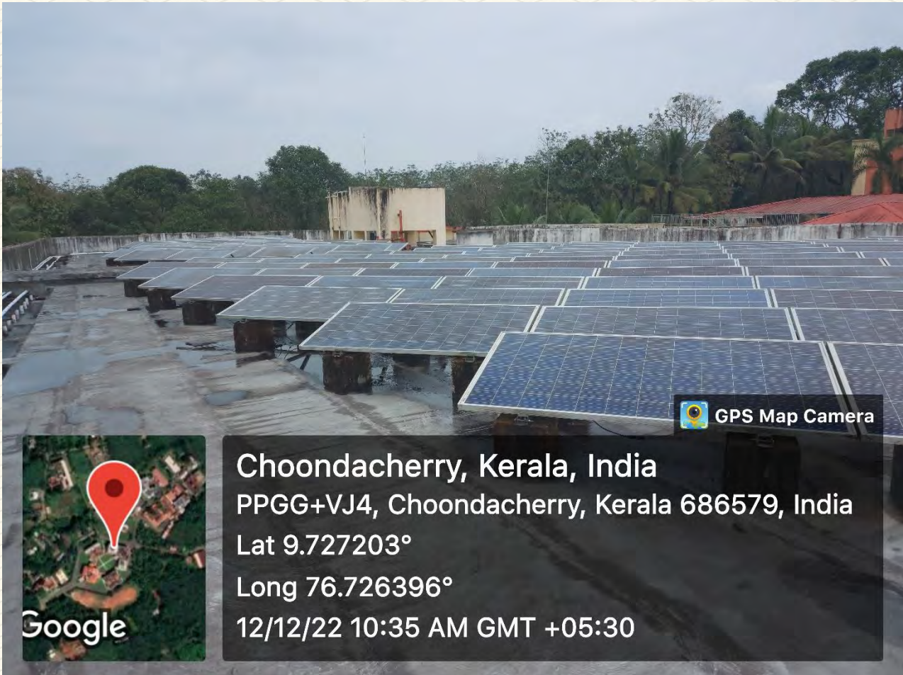
Figure 147: Solar power plant (roof top)
