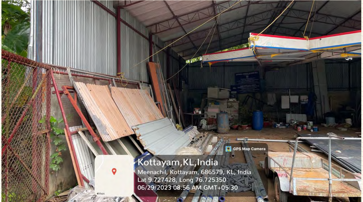
Figure 125: Utility area Photo 2
