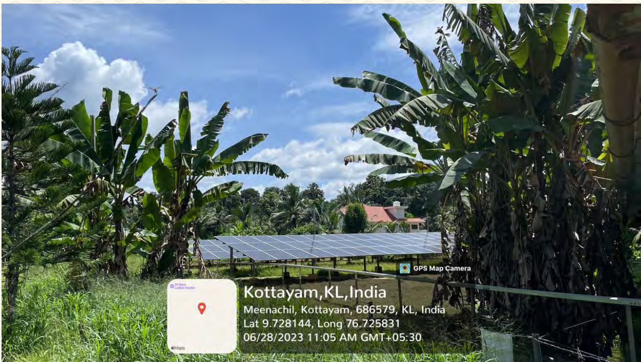
Figure 98: Ground -Mounted Solar Power Plant Photo 3
