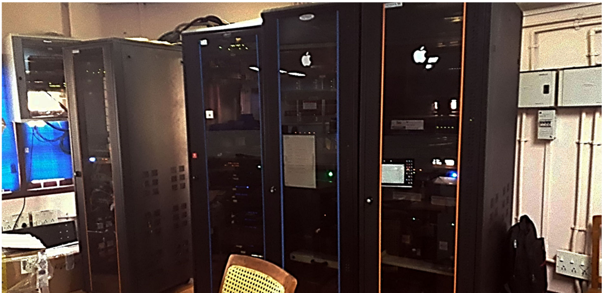
Data Centre – Inside the Server Room
