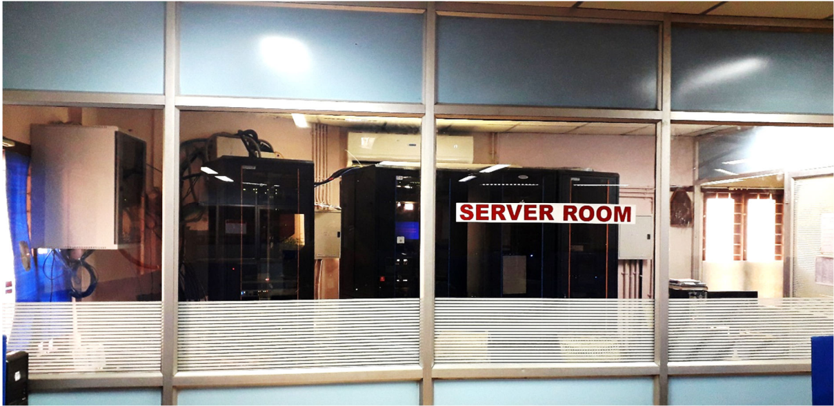
Data Centre - Server Room
