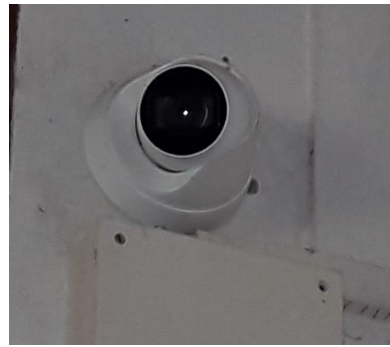
Indoor HD IP Cameras in the Class Rooms
