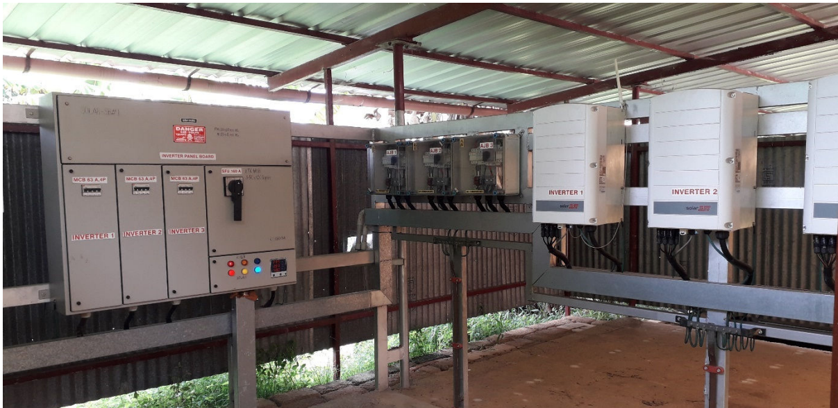
Solar Switching & Metering Station (on-Grid Configuration)
