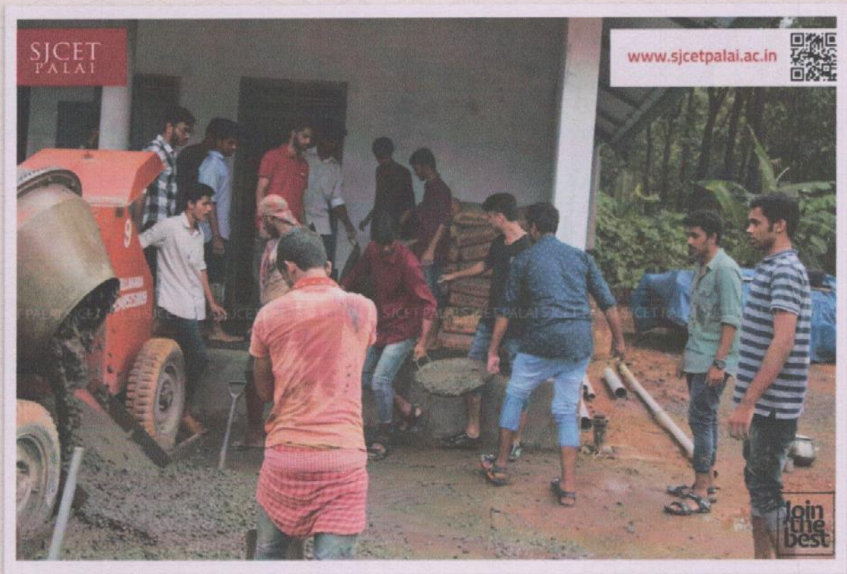
Flooring Work undertaken by NSS Volunteers in Construction of Orphanage at Kuravilangadu during October 2021
