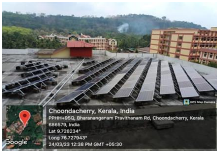
Fig 3. Solar power plant
