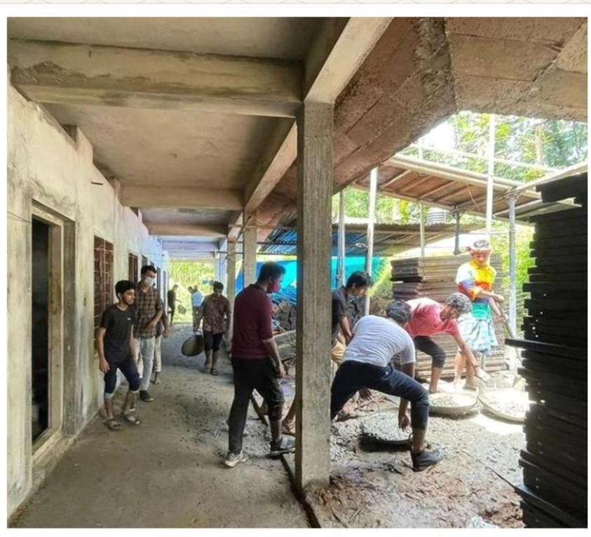
Construction of Old Age Home by Students of SJCET at Manchuvadu, Kuravilangad, 8 th to 10 th October 2021
